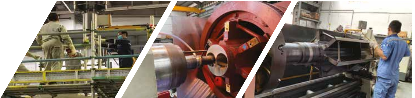
• Rotor Shaft Insertion
